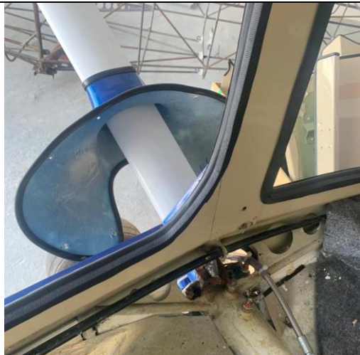
Figura 8 – acabamento do montante (MC01030) desacoplado Figure 8 – Uncoupled wing strut fairing (MC01030)
