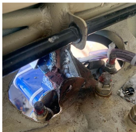
Figura 15 – Peça soldada Figure 15 - Welded part
