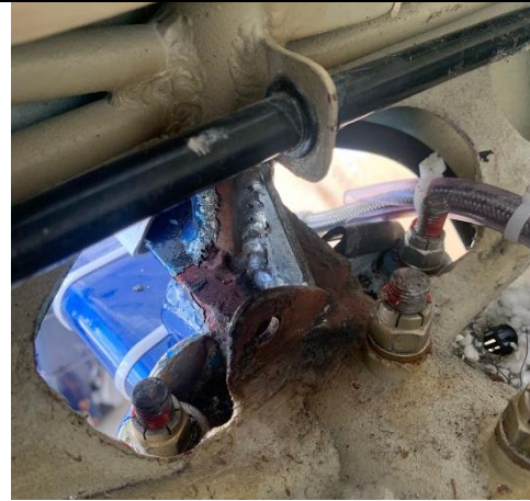
Figura 15 – Peça soldada Figure 15 - Welded part
